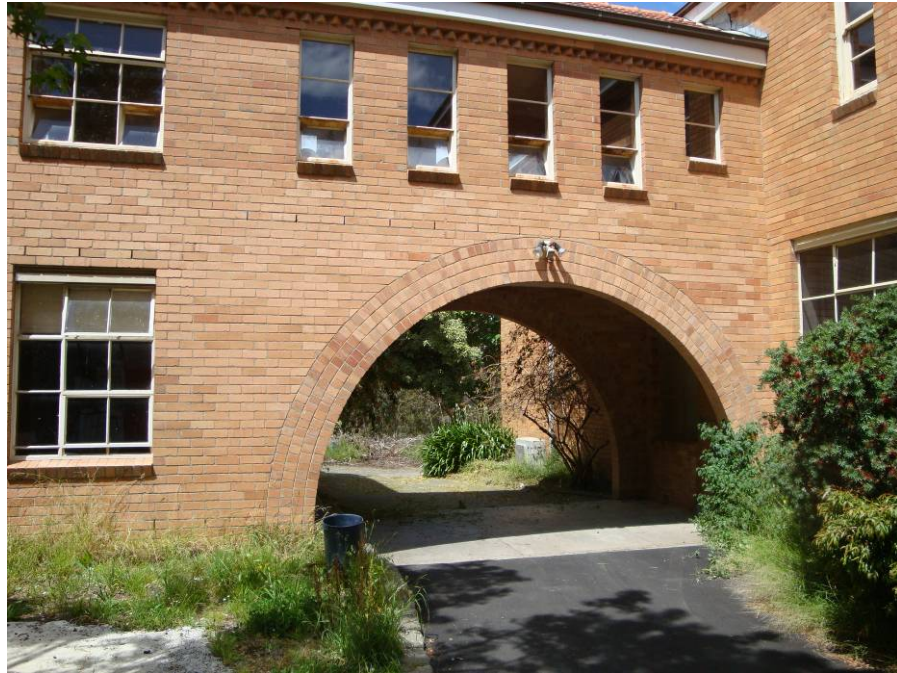
Figure 6: Archway of the 1963 accommodation wing. The bridge that this arch supports connects the wing with the main monastery building.
